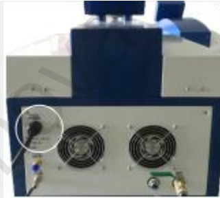
Step 2 Power Line: Red line --firing line Blue line--zero line Yellow line--earth wire
