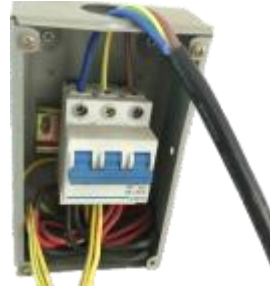
Step 3 put the power line in the switch as step 2
